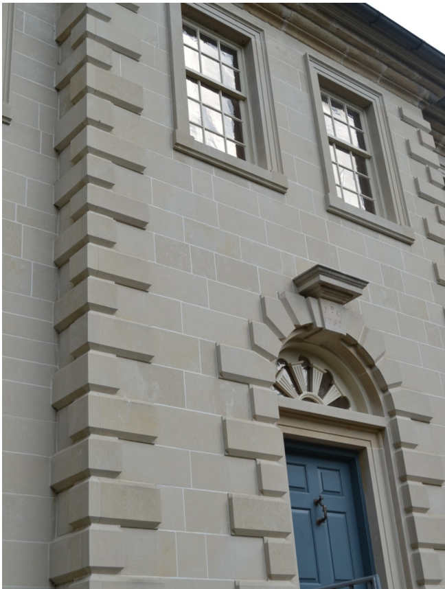
The front façade of the Carlyle House. During the restoration, the house was refaced with Kentucky limestone, which wears better than the local sandstone. Upon close inspection, you can see the original, darker, stone in the cornice.
